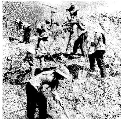
North Vietnamese Workers rebuild a road after a bombing raid, Nghe An province, 1967
